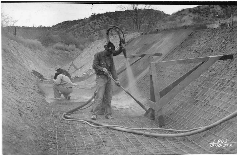
Figure 2. Though here being used to build a canal in 1937, this same method of construction would go on to be adapted for the construction of swimming pools, making them drastically cheaper and faster to build. #294602, U.S. National Archives and Record Administration.
