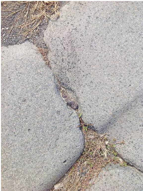
FIG. 3. Example of Type 1, solid without staining, Supplementary Table, ID_044, Via Stabiana (ID = iron deposit). The damage to the paving stones around the iron suggests that the iron was pounded into the junction.
