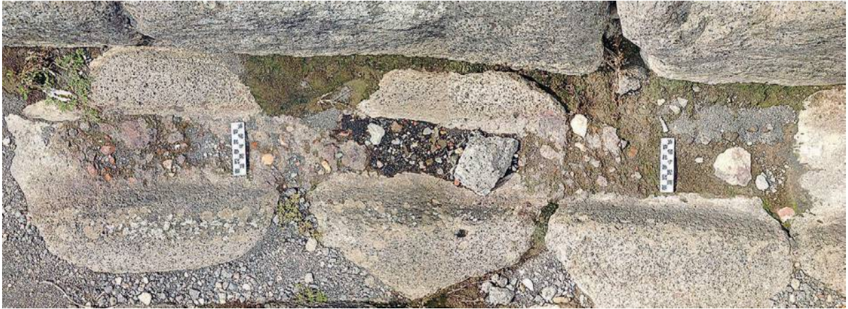
FIG. 15. Example of Type 6, repair with composite materials, Supplementary Table, ID_168, ID_169, Via della Fortuna. Note that the deposit contains ceramics, including terracotta, as well as pieces of marble or white limestone, and it fills only the bottom of the rut.
