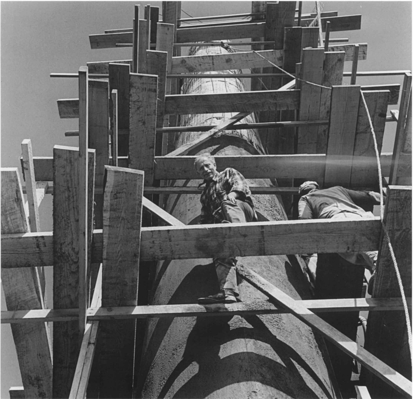
Bufano and an assistant work on a scaffold to rectify the installation of The Expanded Universe (ca. 1970). Bufano's response to the erroneous orientation of the Madonna's head was the installation of a new face of mosaic tile on the statue's east side.
